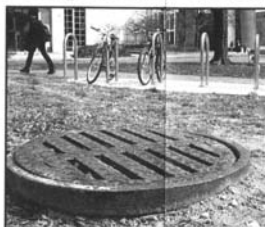
14,000-volt power lines and "an invisible sword" of 600-degree steam: Ohio State says its underground utility tunnels are so dangerous that workers don't enter them alone. Not much. drop 8 feet down into another tunnel.
